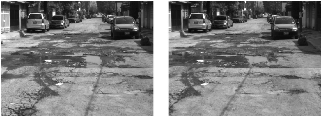
Figure 6.2: The stereo pair “ Street with potholes 1 ”
